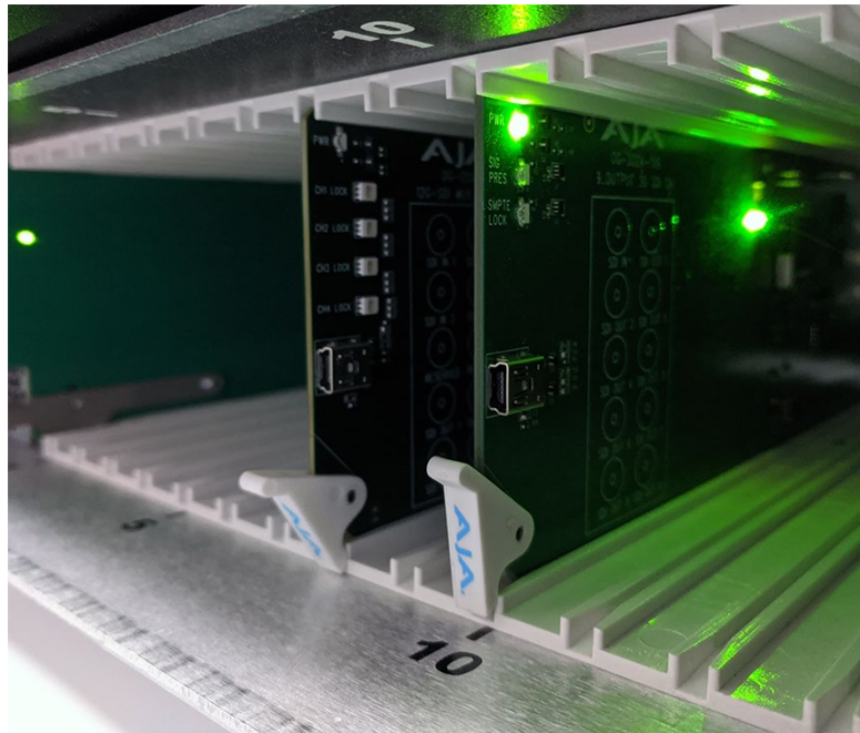
Figure 7. Two OG Cards Inserted into the Frame
