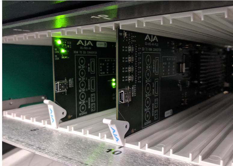
Figure 7. Card on Right Not Fully Inserted
